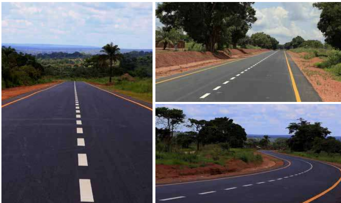
安哥拉北隆达敦多市道路沥青铺设项目 Road Asphalt Paving Project in Dundo, North Lunda, Angola
