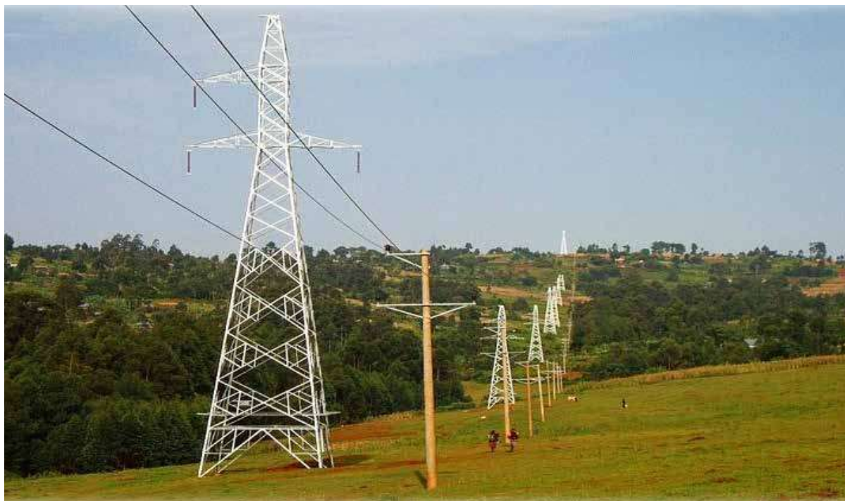
肯尼亚电网改造一期 The Kenya Power Distribution System Modernization And Strengthening Project Phase I
