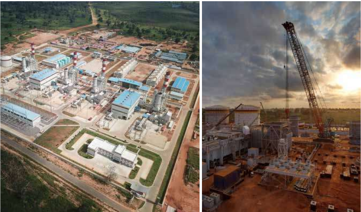
安哥拉索约联合循环电站建设与安装项目 Construction and Installation of the SOYO I Combined Cycle Power Plant Project in Angola
