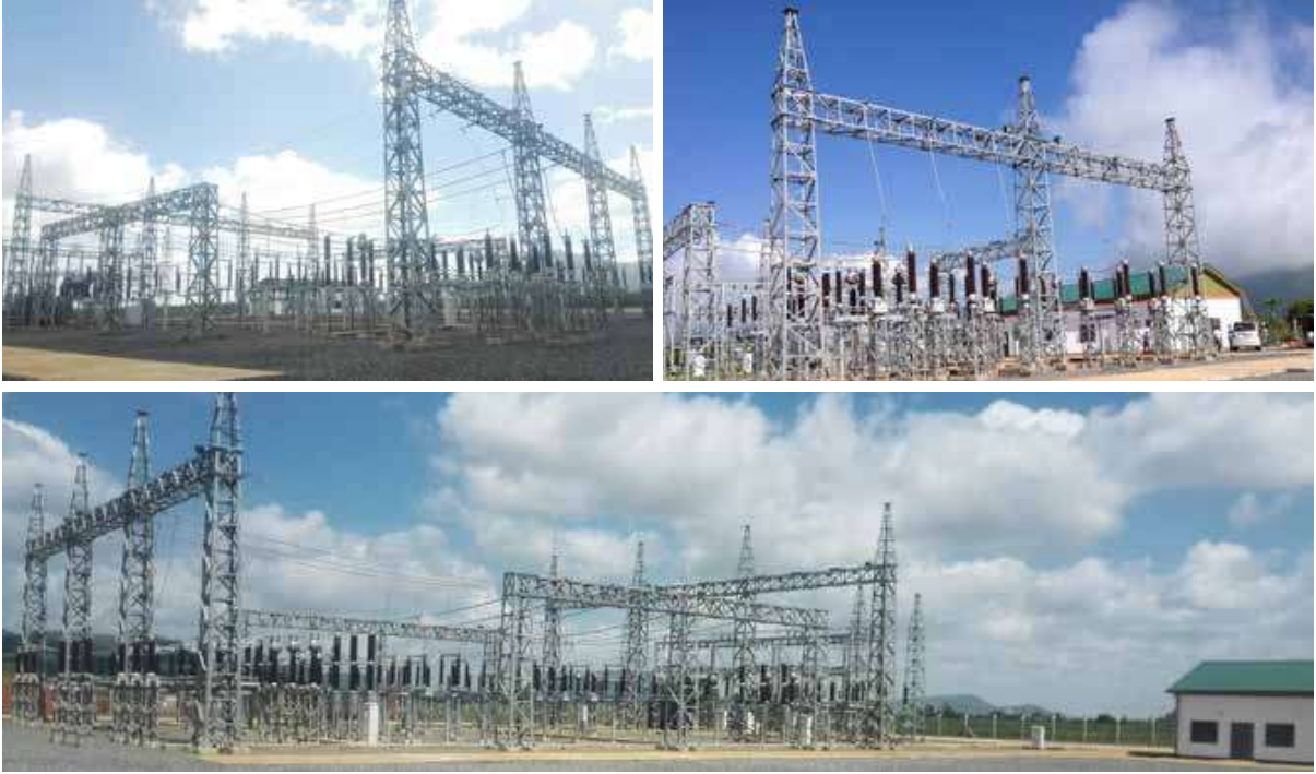
肯尼亚电力传输系统升级改造项目 LOT3B Kenya Power Transmission System Improvement Project Lot 3B
