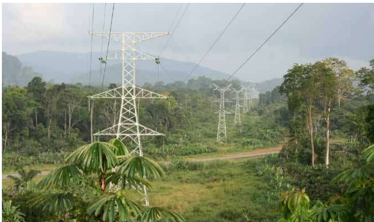
非洲西部最大最稳定的国家电网—赤道几内亚吉布劳水电站输变电项目 Africa's largest and most stable national grid-Transmission Line and Substations for Djiploho Hydro Power Station Project
