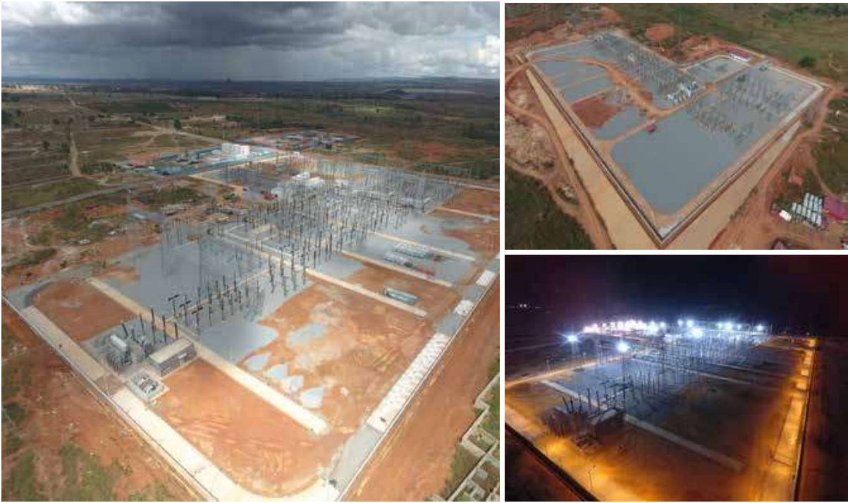
安哥拉 LAUCA 连接线项目 Transport System Associated With Lauca (Lauca-Huambo) in Angola
