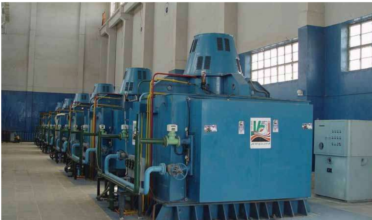
苏丹桑多斯泵站项目 Sondos Pumping Station in Sudan
