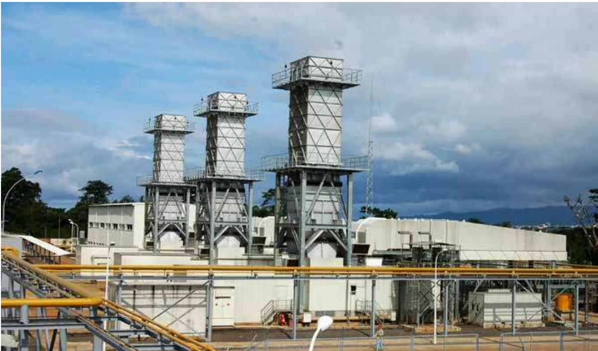
赤道几内亚马拉博欧洲角电厂扩建项目 Malabo Gas Turbine Power Plant Extension Project in Equatorial Guinea
