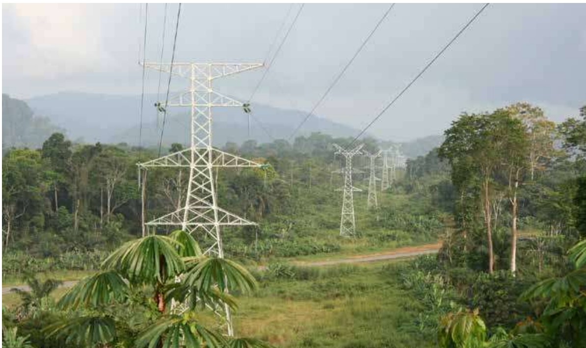
赤道几内亚吉布劳水电站输变电项目二期工程项目 Transmission Line and Substations for Djiploho Hydro Power Station Project (Phase II) in Equatorial Guinea
