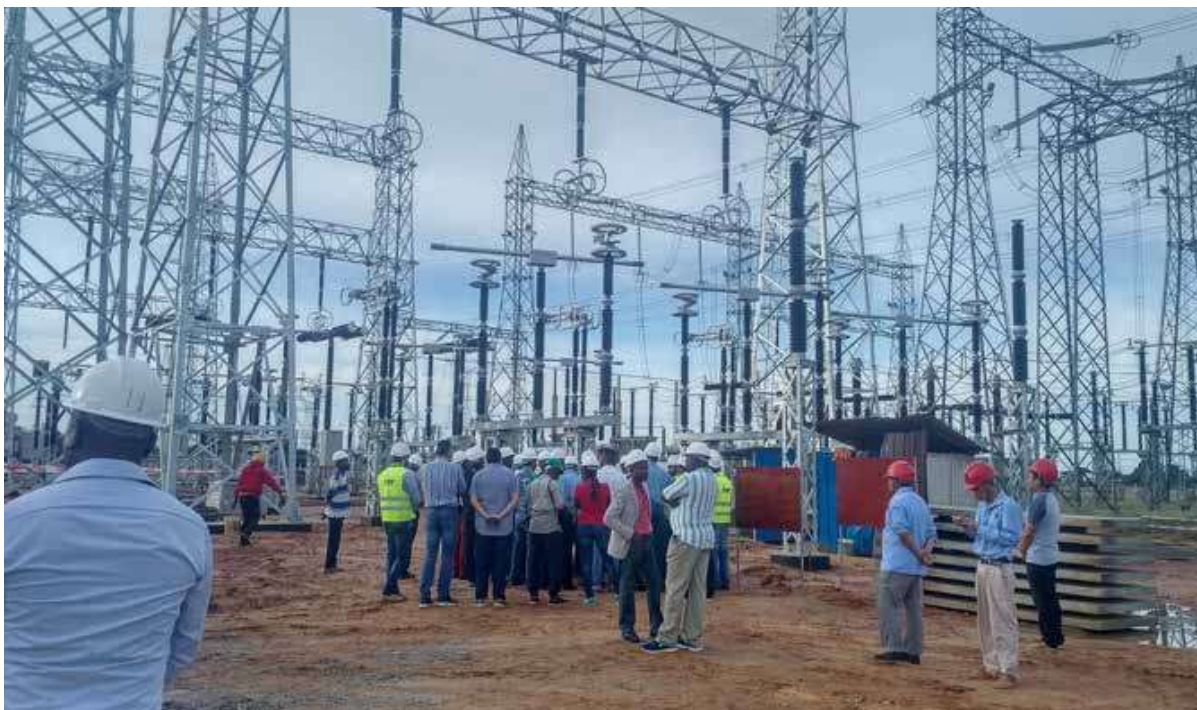
建设罗安达地区索约电站连接线项目 Construction of Associated Lines with Soyo Combined Cycle Power Plant Project in Angola
