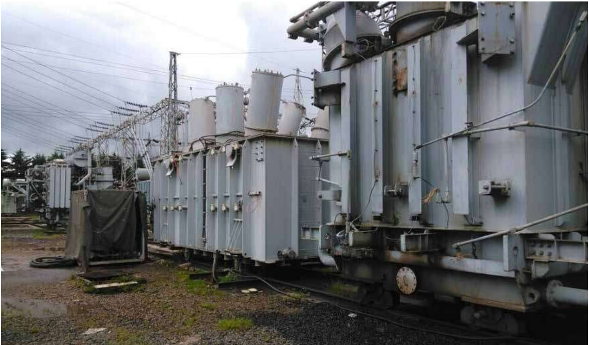
埃塞伯代莱 - 默图电力输变电工程 230kV 输电线路材料的供货项目 (BM-2) Bedele-Metu 230kV Power Transmission Project in Ethiopia Contract BM-2 Supply of Transmission Line Materials
