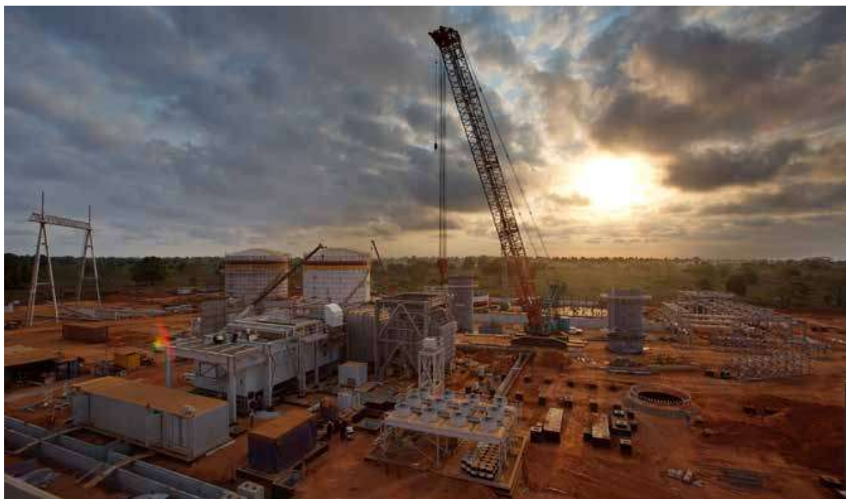
非洲最大燃气轮机电站—安哥拉索约联合循环电站 Africa's largest gas turbine power station - SOYOI Combined Cycle Power Plant Project in Angola
