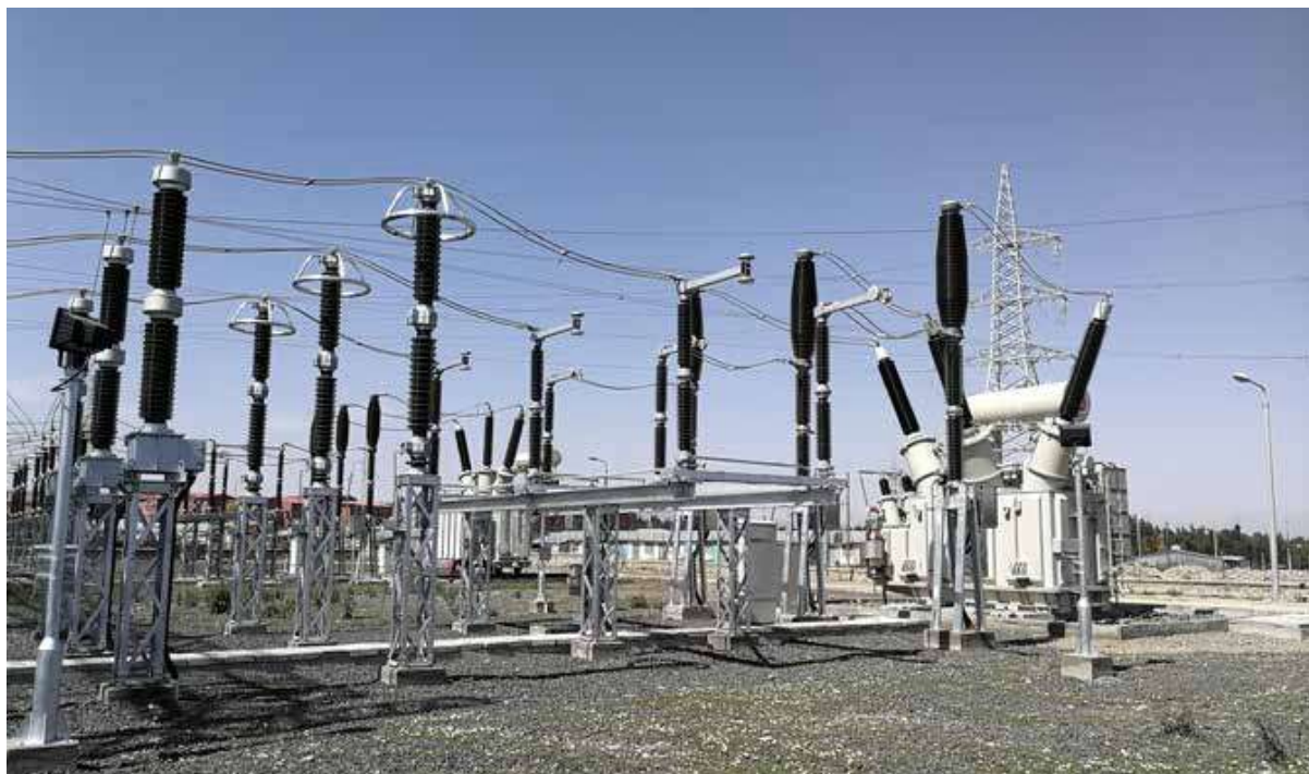
埃塞 Contract-H 变电站扩建项目 Lot2 Electricity Network Reinforcement And Expansion Project (ENREP), Transmission And Substations Rehabilitation And Upgrading Component Contract-H in Ethiopia
