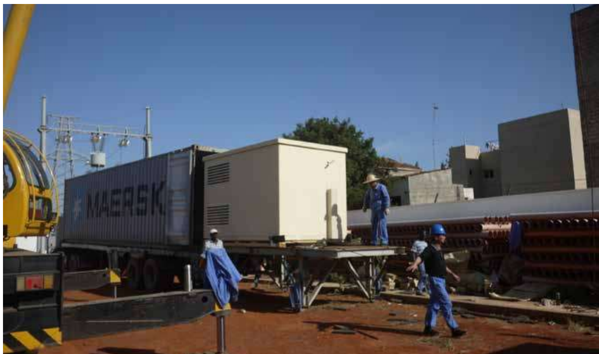
塞内加尔达喀尔配电网改造及扩建项目 Project Extensions and Rehabilitation of Networks in Dakar in Senegal
